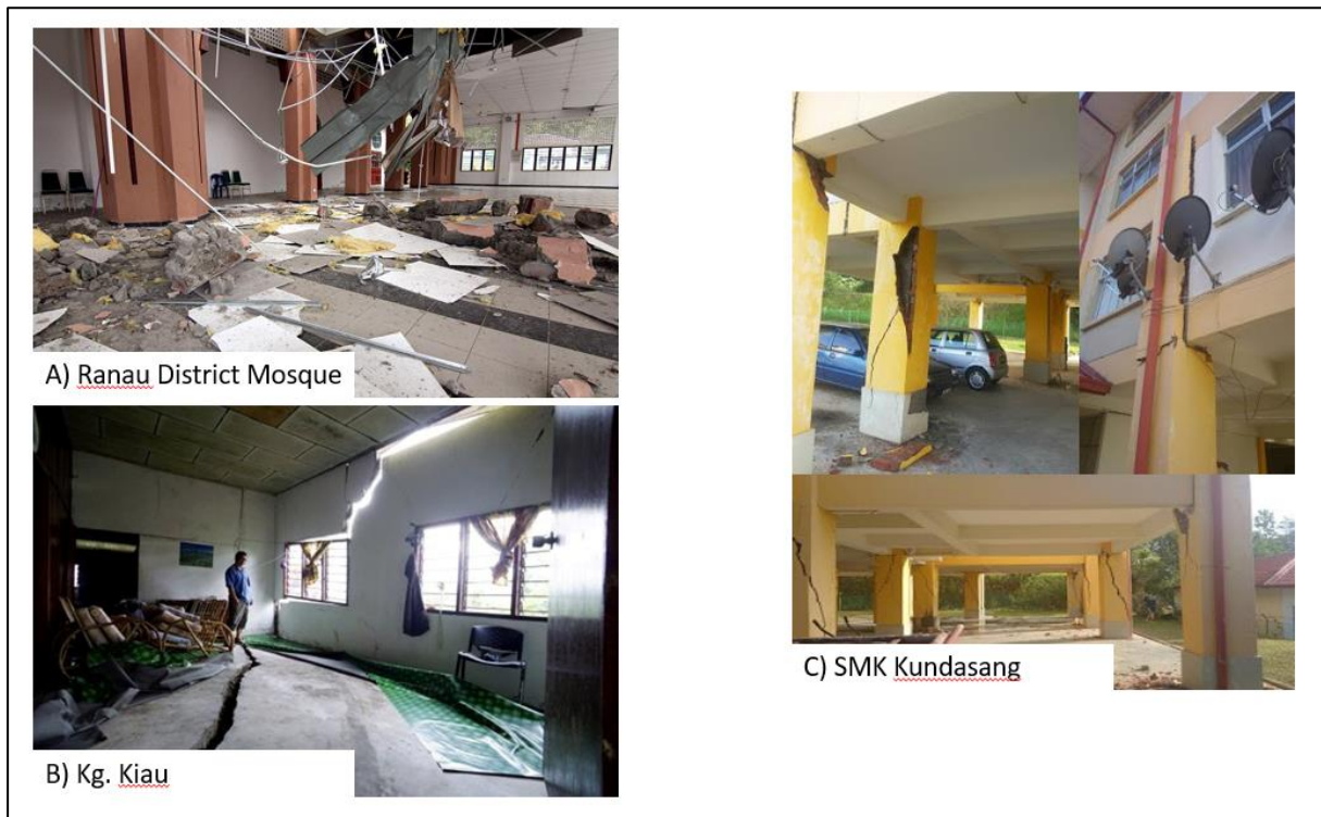
Figure 2. Situation in some places of the study area affected by the earthquake.
