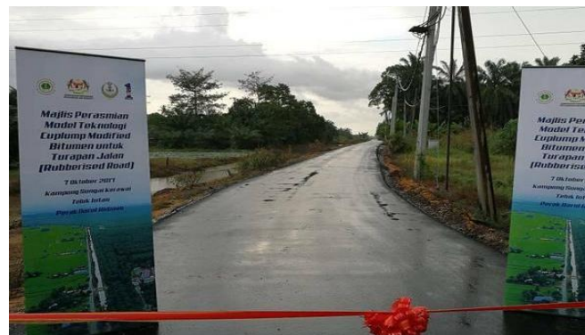
Figure 7. Ciplump Modified Asphalt (CMA) road along Sungai Kerawai in Teluk Intan, Perak [48]
