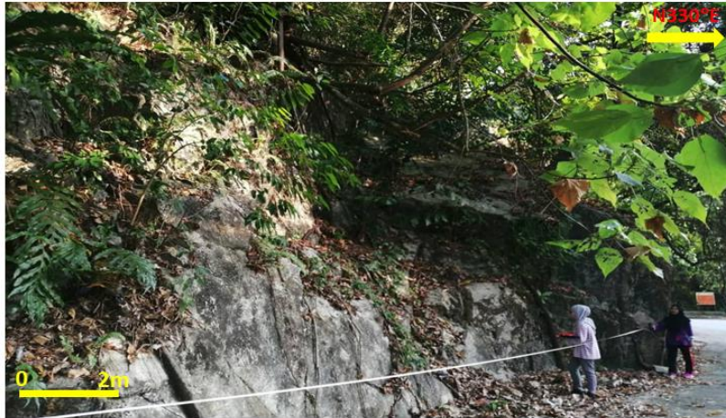
Figure 2. The outcrop of study area is beneath Grandview Heights. The scanline method was conducted to quantify the discontinuities of the rock mass forming the slope.
